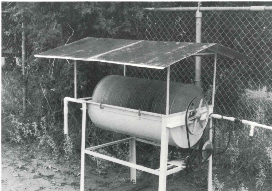
The small rotating biological contactor above was built by NMSU's Civil, Agricultural and Geological Engineering Department and is now being used to treat the septic tank effluent from three mobile homes.
